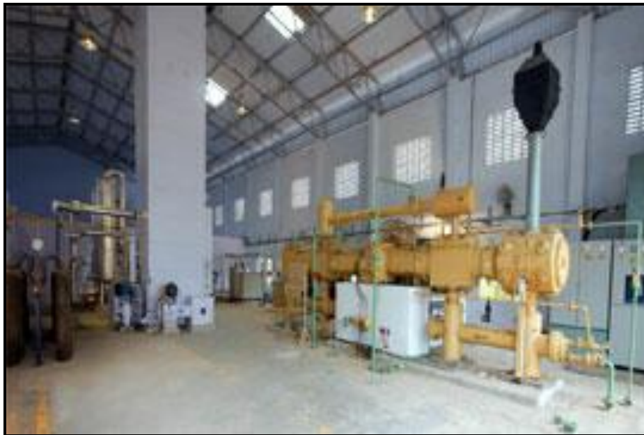
Figure 8-3: Air compressor for Oxygen Plant
