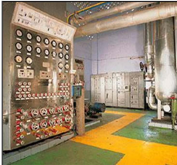
Figure 8-1: 300 m 3 /hr. Plant View
