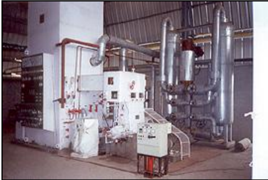
Figure 8-2: 300 m 3 /hr ASU & Expansion Engine and M.S.B
